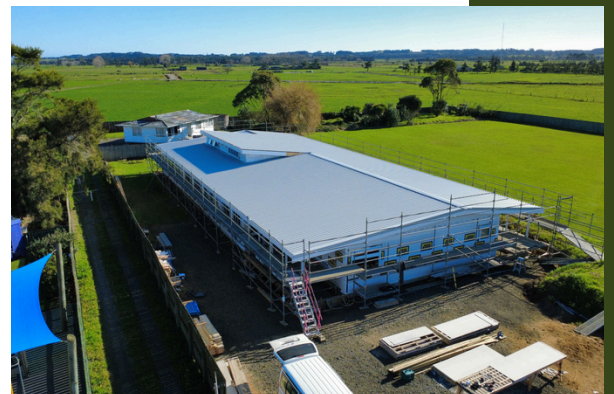
Blomfield Satellite School Construction
